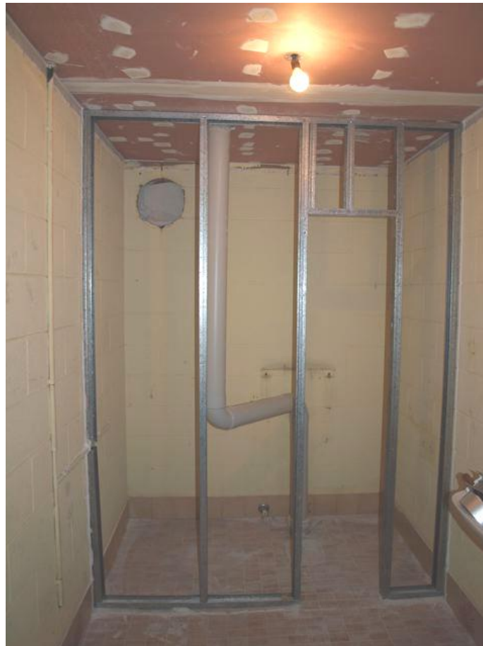
Figure 3.2 Pipework in Test Rooms
