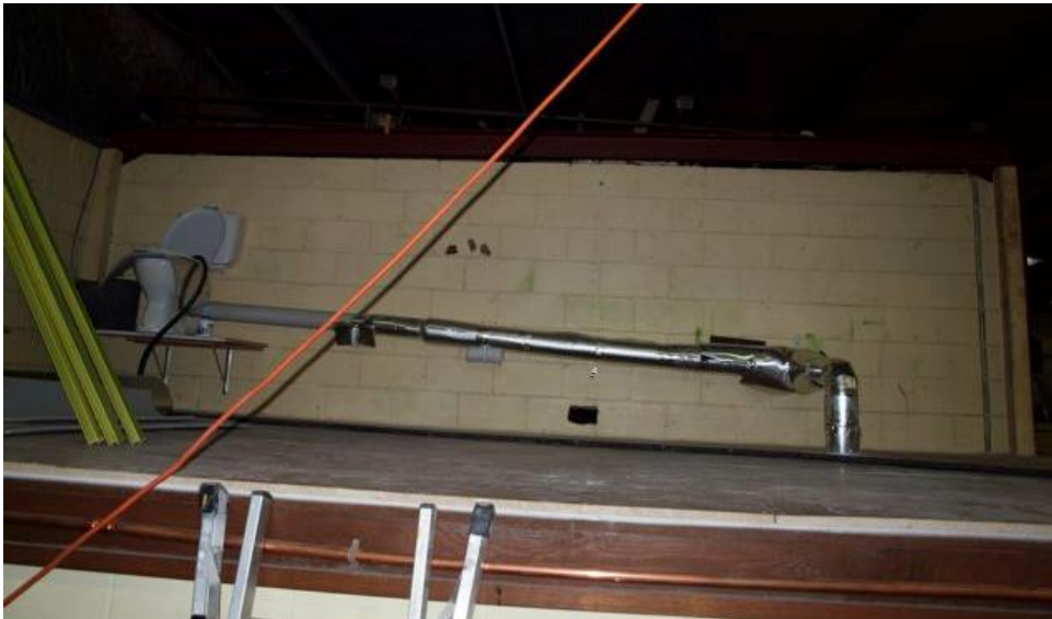
Figure 3.5 Cistern and Pipe above Test Rooms
